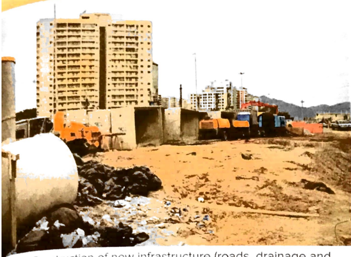
3.80 Construction of new infrastructure (roads, drainage and housing) in the Barra district as part of the Olympic Games preparation.
