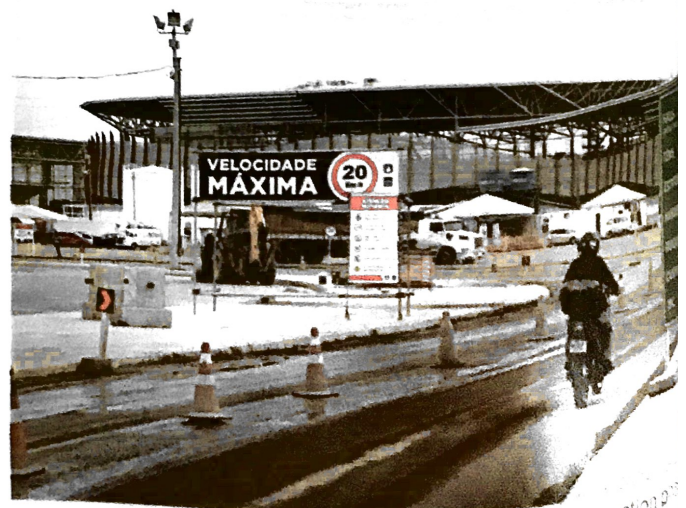
3.79 The Barra Olympic venues during their construction one year before the Games (in July 2015).
