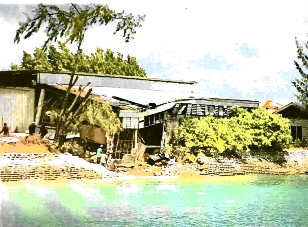
6.21 The seawall at Betio Harbour was breached by wave attack during a storm, allowing waves to intrude and erode the coral sand foundations of this factory. As the sand was eroded, the factory partially collapsed.
