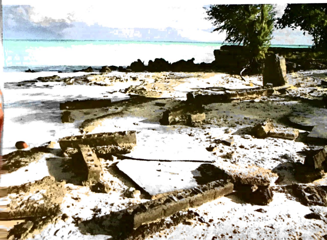
6.22 This house in Bikenikora village was destroyed by wave attack after the seawall that was built protect it from wave attack was undermined and destroyed. The remains of the seawall can be still seen in the background.
