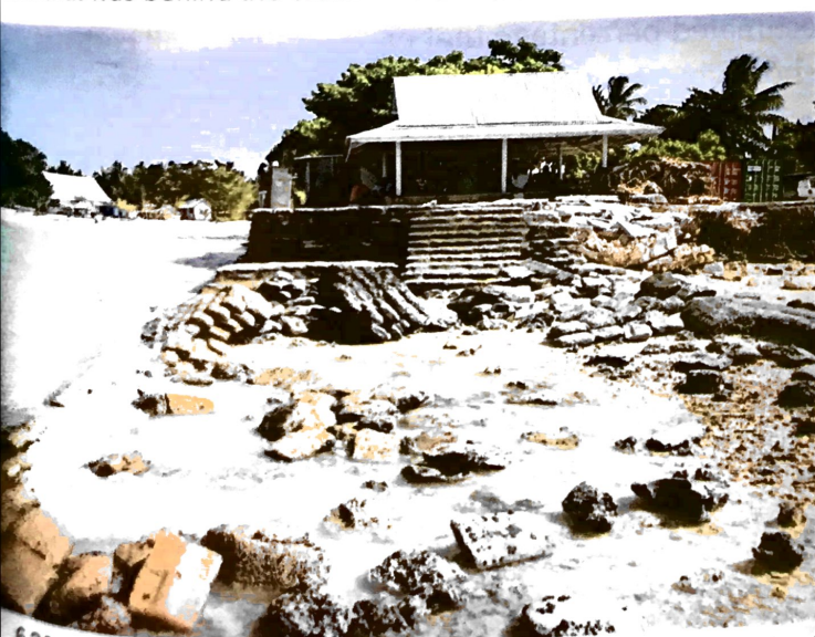
6.30 This seawall at Bairiki has been almost completely washed away, allowing the ocean water to inundate land that was previously about one metre above sea level.
