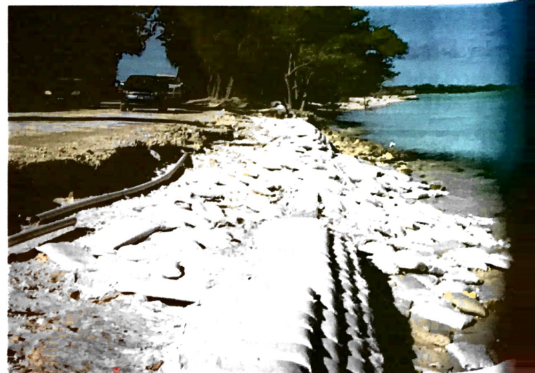
6.28 Wave action has undercut a sea wall that was protecting the main road between Bonriki and Bairiki.
