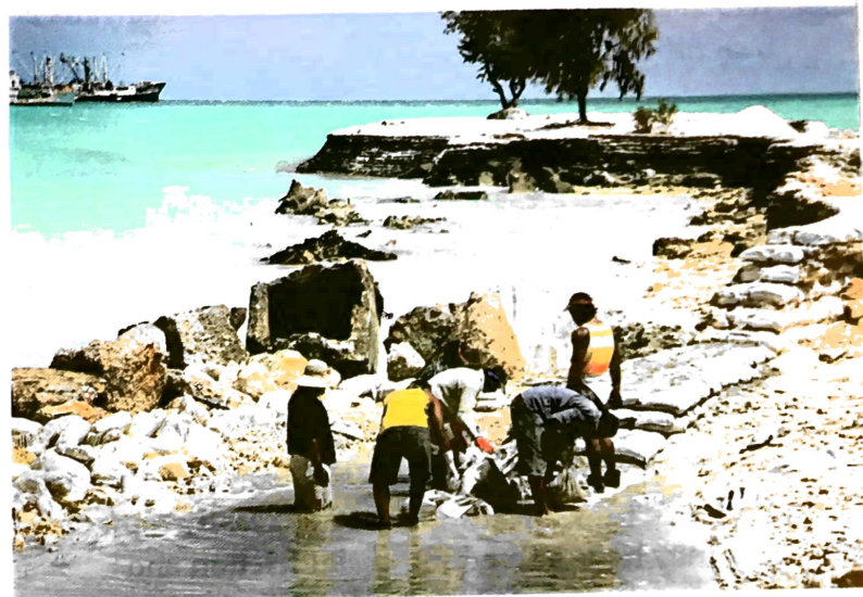
6.31 Workers repair a section of seawall that has been undermined, forcing it to collapse near Red Beach, Betio Island.
