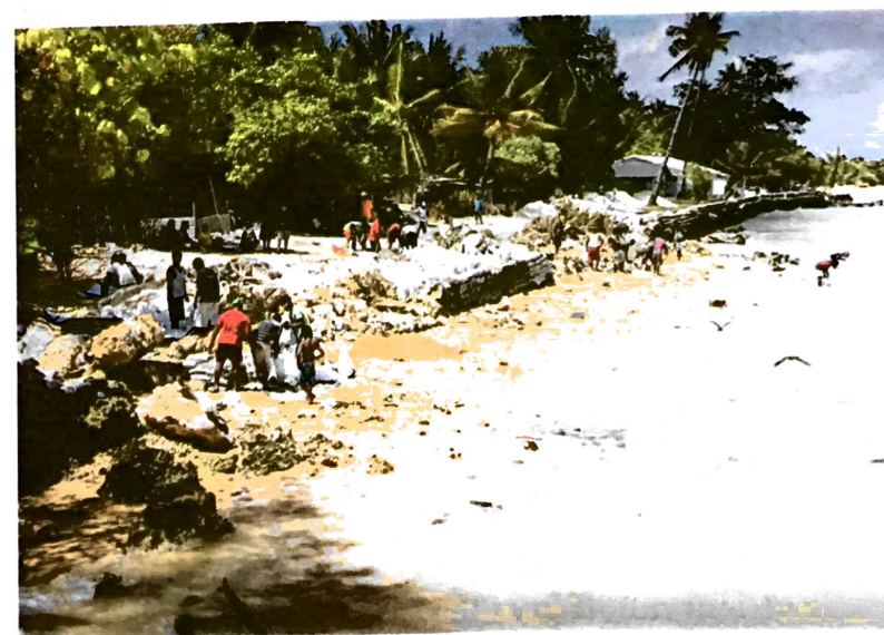
6.32 A large section of seawall has collapsed in the face of wave attack, and a large group of about 30 workers is filling bags with sand before sealing the bags and cementing them in place to build a new seawall.
