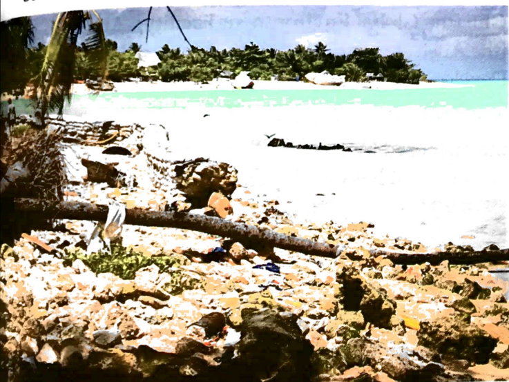
6.29 This seawall on the northern side of Betio Island has been washed away, allowing waves to erode a substantial area of land that was behind the wall.
