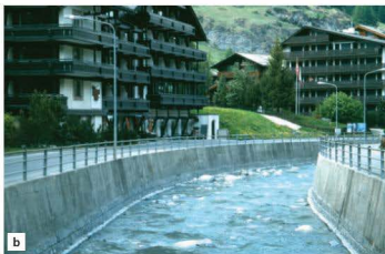
Figure 25 Hard engineering structures a River defences - River Thames in London b Levées in Zermatt, Switzerland
