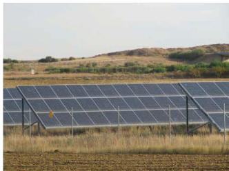
Figure 12 Solar electricity being generated by photovoltaic panels in Spain
